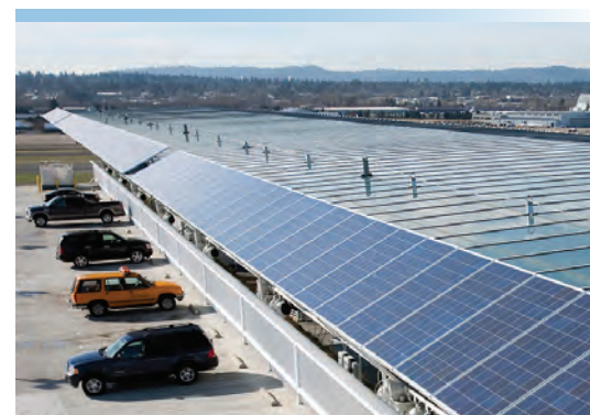
Nike, Delta Air Lines, and the Port joined forces to install solar panels on the Airport's canopy
